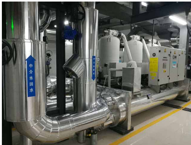
Figure 24: Heat pump in Uni Town. Photo credit: City of Qingdao.
